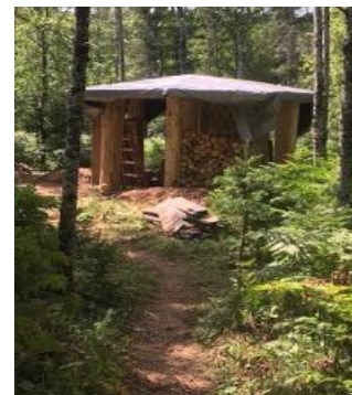
Construction of the roof for the eight sided building was the work that took the most time (and head scratching), but it was finished and covered by August 13th.... Ready for cordwood walls to go up!
