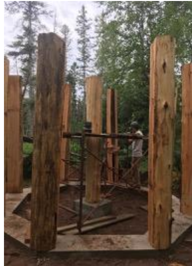
July 24th and 25th: nine large cedar posts were brought in to the site on foot and erected at the corners. This was the work requiring the most muscle, and 7-8 strong men rose to the occasion! Seen here: Rich Sloat, Jonny Waara and Brody Eckburg. Not pictured: Tom Coats, Gary Pisoni, Terry Yackel, Jon Ahlberg.
