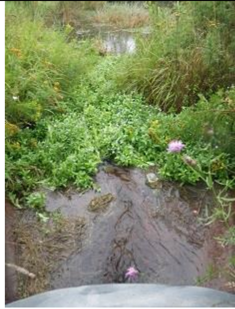
Fig. B-20. SC239, stormwater outfall to pond adjacent to Iron River, facing downstream. 20 August 2016. .
