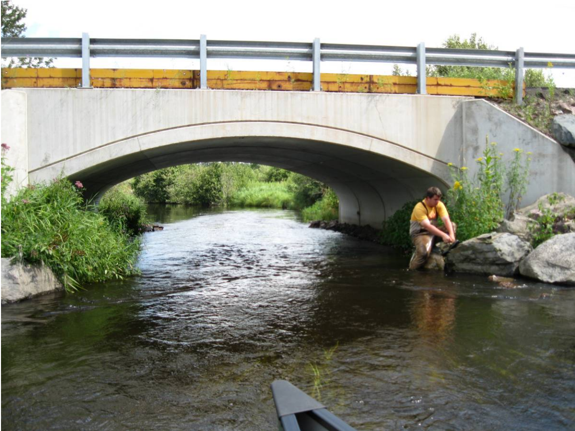
Figure 32: The Mottes Rd culvert, a great example of a bottomless road crossing that does not act as a bed control on the stream slope and passes aquatic species easily. This crossing does cause a flow constriction and ideally should have been sized for slightly wider than a bankfull width, but the impact is minor.
