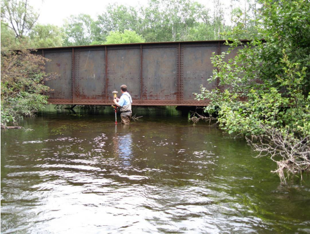
Figure 44: Several low bridges, relic RR crossings now used for the ORV trail are within the reach. These don't appear to have an impact at normal flows, but likely back up water during flood flows. The condition of these bridges indicates they are near the end of their design life. Replacement structures should be built within a restoration context of the reach and ensure little impact on river transport and fish passage.
