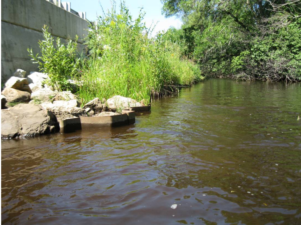
Figure 49: Brady Ave crossing, showing some armoring of the stream bank with sheet pile.
