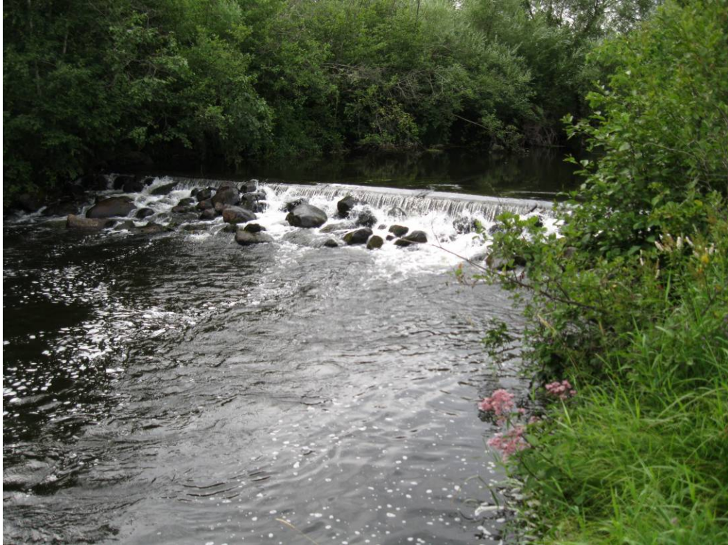
Figure 47: The dam at station 37,700 is blocking fish passage but is an integral part of a wetland remediation project upstream. The dam should be removed and could be replaced with a series of riffles to accomplish the same purpose and improve habitat.
